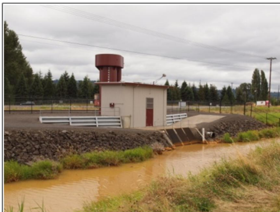
Photo 1: Oregon Way Pump Station
