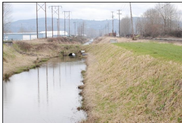
Photo 2: View of CDID Ditch No. 3 on the east side of Oregon Way, looking east
